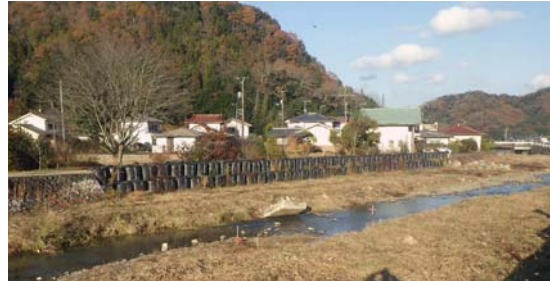
▲被災後応急復旧
